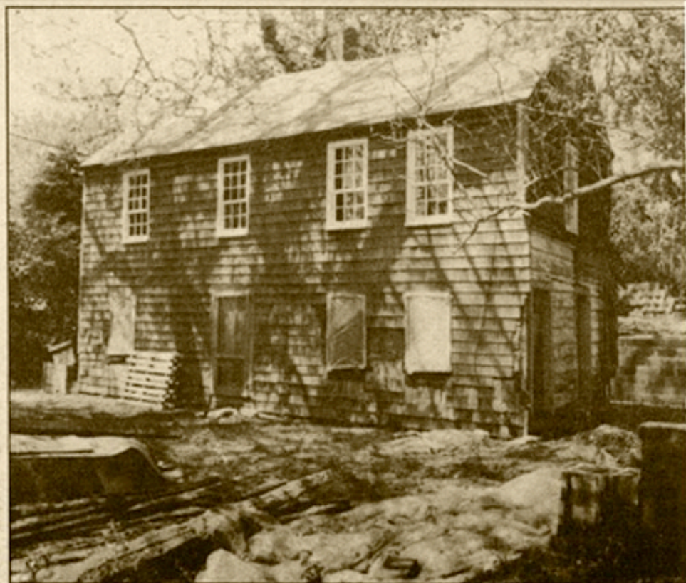
After only five years in business, Peter Stoutenburgh, top, now employs more construction workers at Environment East than any other North Fork builder. The company, best known for its rehabilitation work, is making this 1655 structure livable without sacrificing authenticity.
